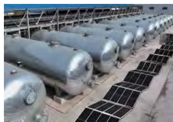
Seawater Treatment Plant
