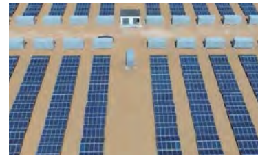
Ground Power Station
